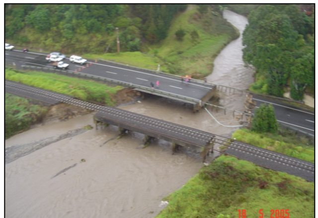
Figure 5: Pikowai Bridge SH 2 RP 209/3.040 - Photo taken at 10:00hrs 18th May 2005. (Source: Transit NZ – Hamilton Office)
