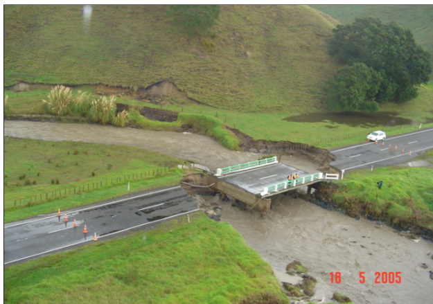
Figure 4: Hauone Bridge SH 2 RP 209/3.040 - Photo taken at 10:00hrs 18th May 2005. (Source: Transit NZ – Hamilton Office)
